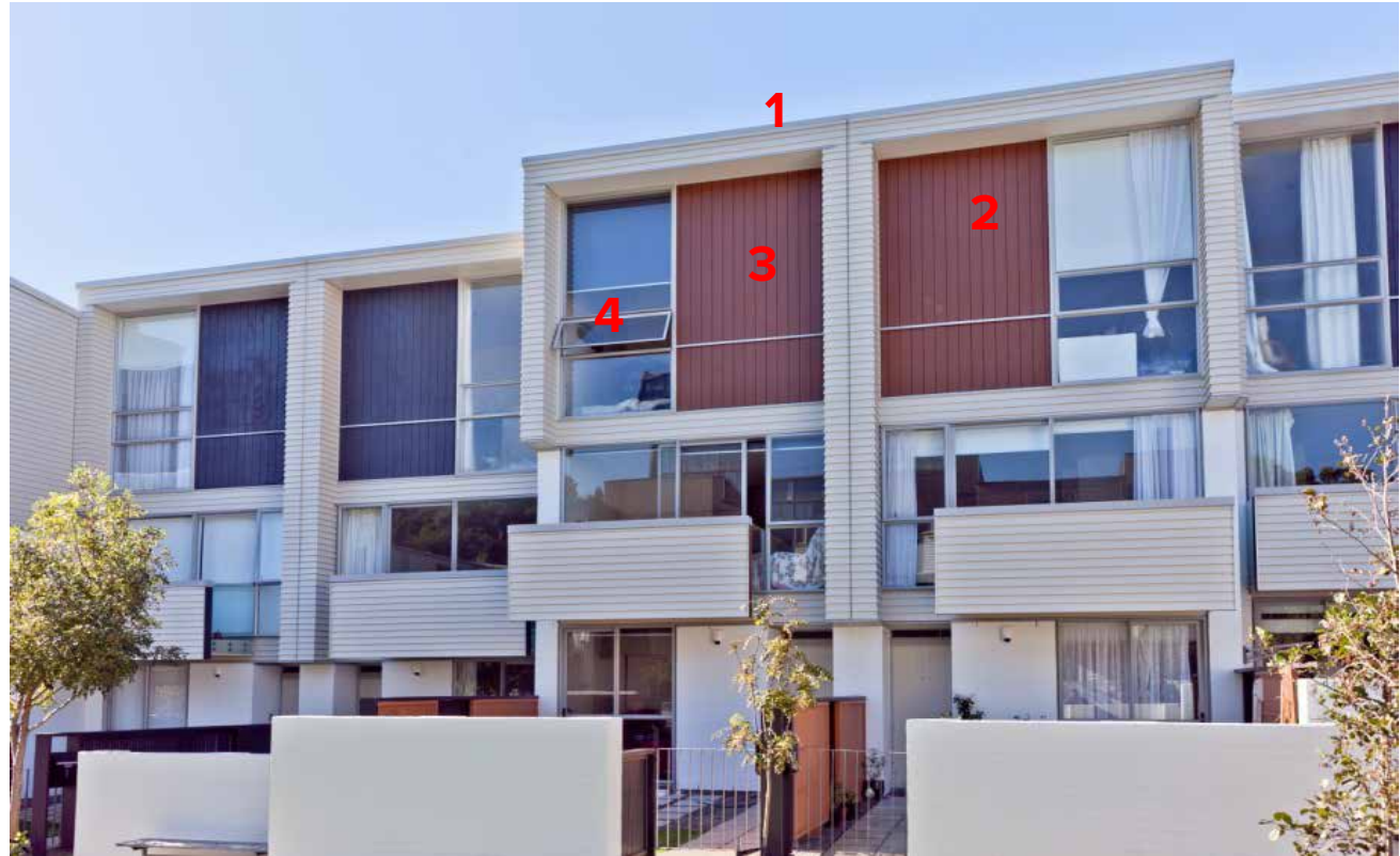
Looking closer at the western elevation of the front terrace block – view from internal communal open space.
