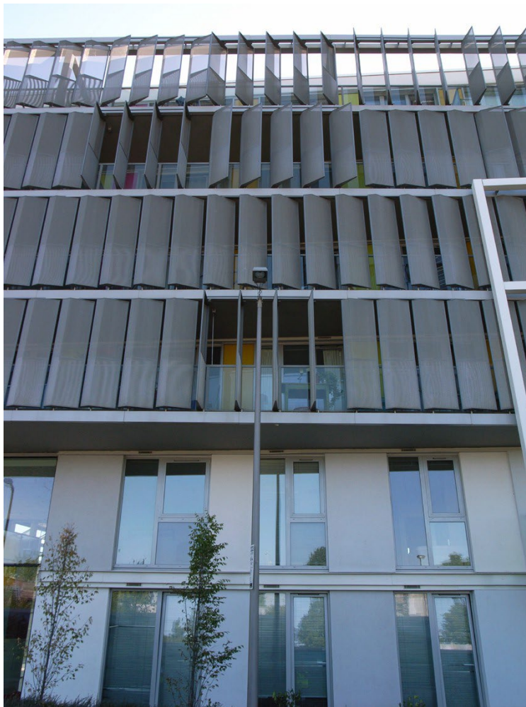
Rotating vertical louvres allow residents to modify and reduce passive solar gain.
