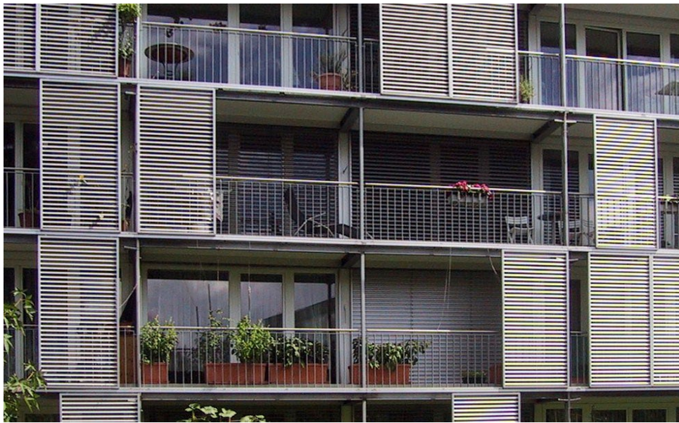
The movable screens in this building are located on long tracks. This means the whole façade changes on a regular basis as the residents move their individual panels as they need them.
