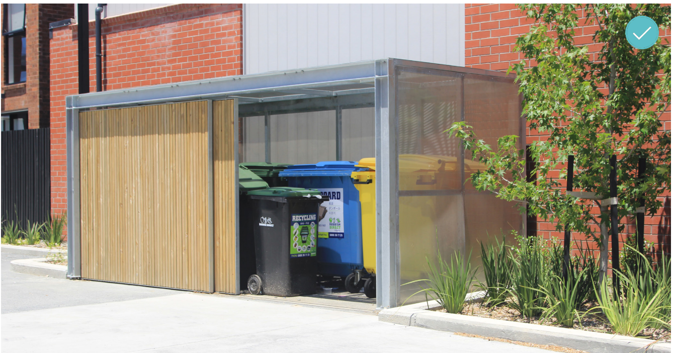
Communal waste bins are stored in an attractively designed, easily accessible communal waste area. Access is via an easily operable sliding door. The walls of the storage area provide good levels of ventilation, but could be opaquer to lessen the visibility of waste bins.
