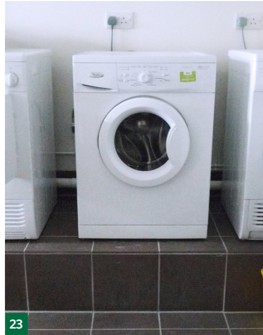
Washing machines and dryers on a plinth in a laundry room.
