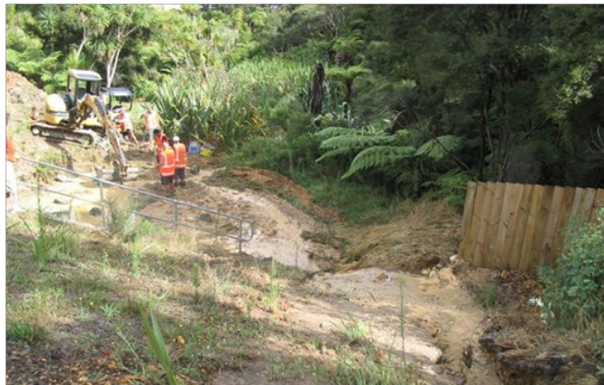
Figure 13: Sediment discharge as a result of not protecting the watercourse
