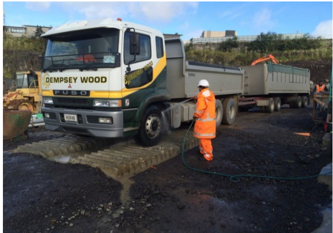
Figure 37: Example of truck wash and shaker ramp
