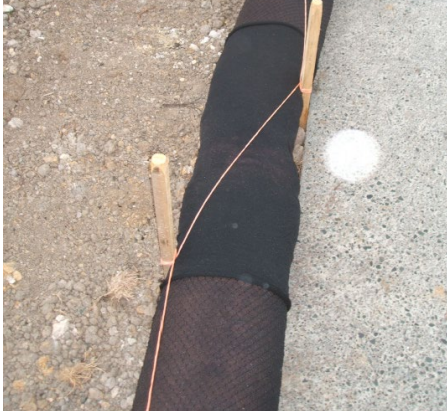
Figure 93: Silt sock joined using a sleeve and pegged and secured using bailing twine with 1 m overlapping joint
