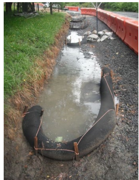
Figure 27: Silt socks can be used as a check structure on a low gradient channel
