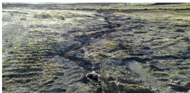
Figure 47: Loss of topsoil and grass seed after heavy rain event. Will require stabilisation and reapplication
