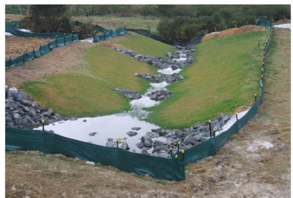
Figure 26: Check dams installed in series to act as a permanent water velocity control measure
