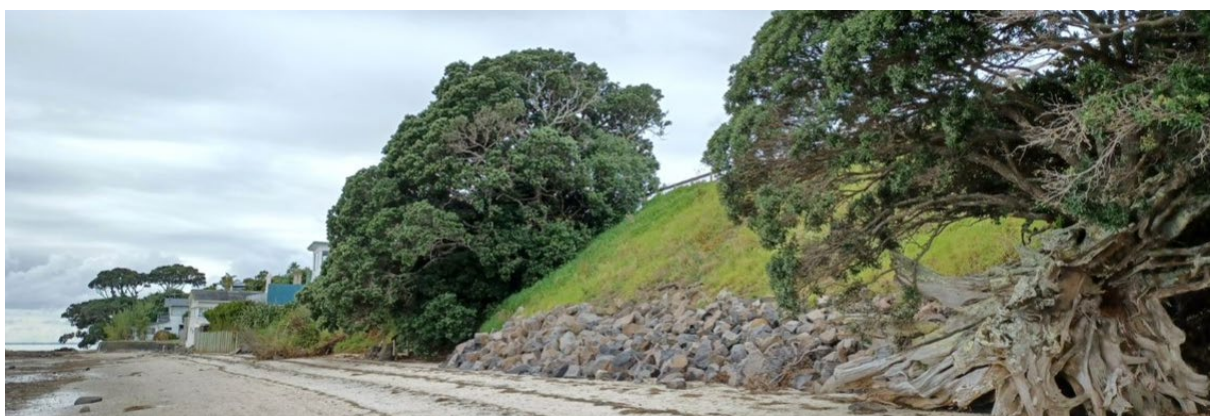
Figure 5-21: Cliffed section of road reserve showing a rock revetment installed in response to a coastal landslide
