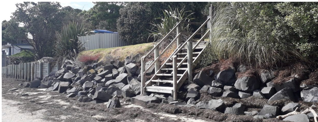
Figure 5-26: Existing timber stairway proving public access to the beach at Hoskings access
