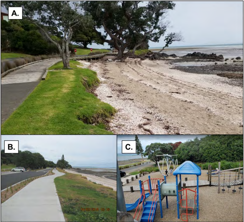
Figure 21: Photographs of western end of Ōmana Esplanade showing on-going erosion (A), eastern end of Ōmana Esplanade along the carpark area (B), and playground facilities in Ōmana Esplanade Reserve (C)
